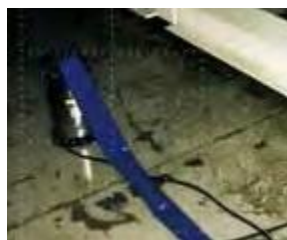
Small drainage pumps
